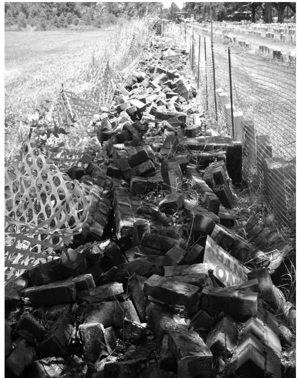
Figure 13-1. Damaged cemetery walls at Chalmette, 2008. (author)
